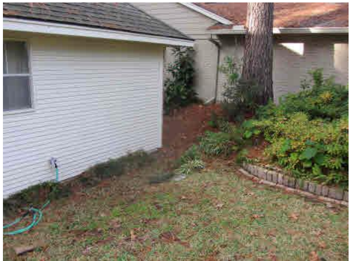
REAR VIEW OF THE MASTER BATHROOM: NOTE THE HIGHER GROUND RIGHT BEHIND THE HOUSE IS THE FAULT ZONE
