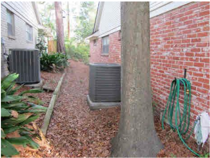
LEFT SIDE OF HOME: NOTE THE HOME ON THE LEFT (13634 PINEROCK) IS MUCH HIGHER THAN THE SUBJECT.
